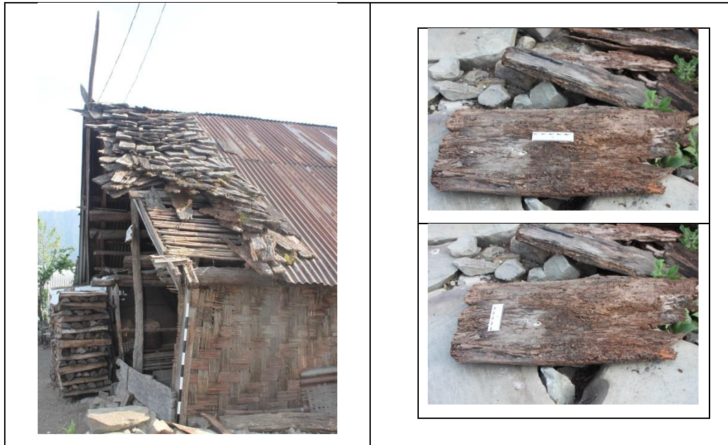
Plate 96: A priest's house in Zhavame village, Phek district, remains partially constructed with wooden planks and fallen pieces serving as a surviving testament.
