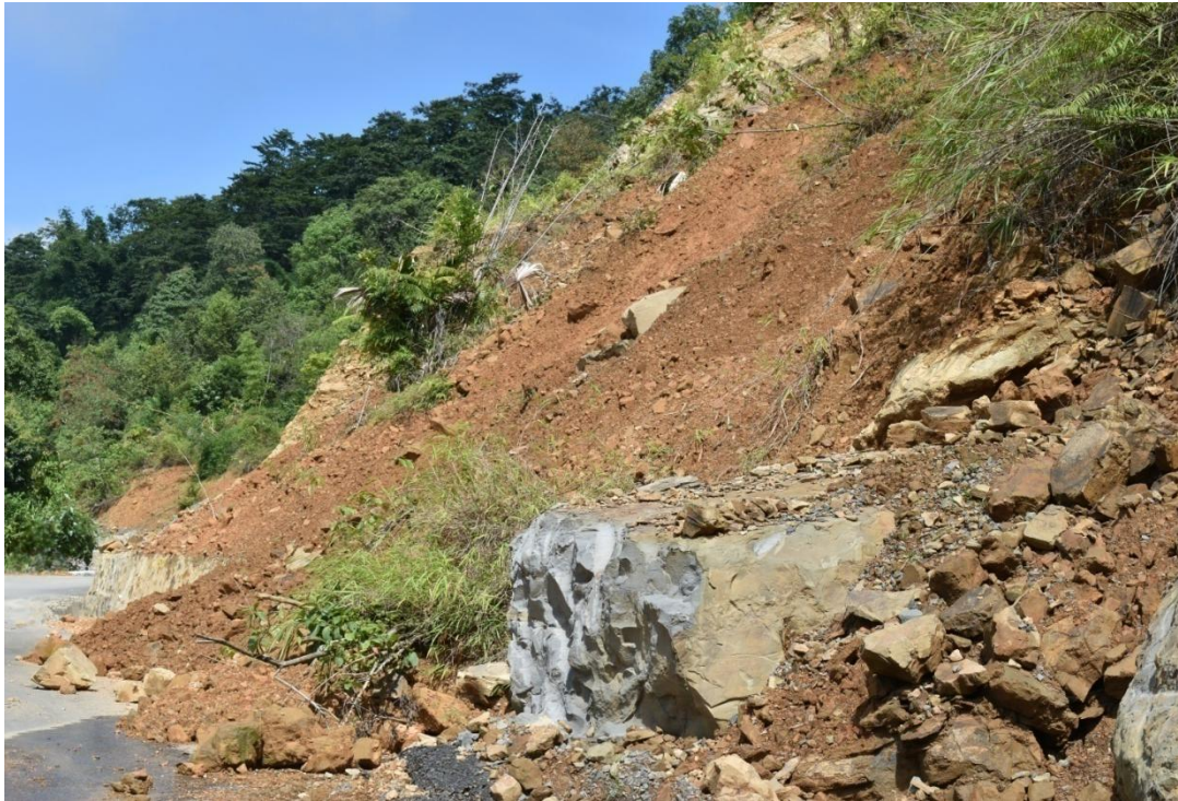
Plate 5.3: Field observation of road cutting related slope failure illustrating weakened slope structure, loose debris and signs of continued mass movements.
