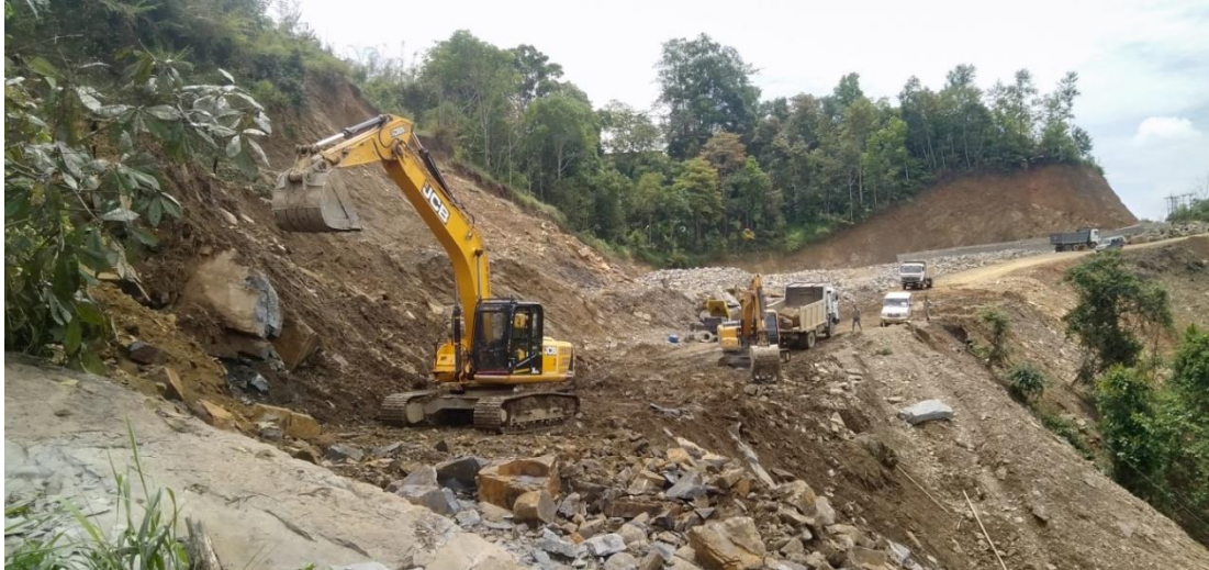
Plate 5.1: Rock Debris along a road cut, indicating shallow slope failure triggered by excavation and rainfall.
