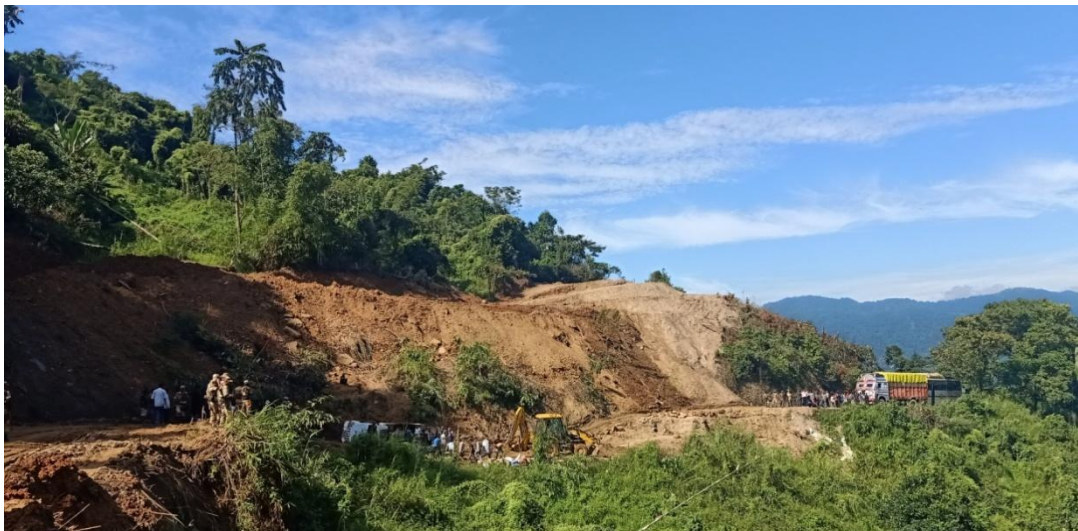
Plate 5.4: Subsidence related slope failure affecting road infrastructure.
